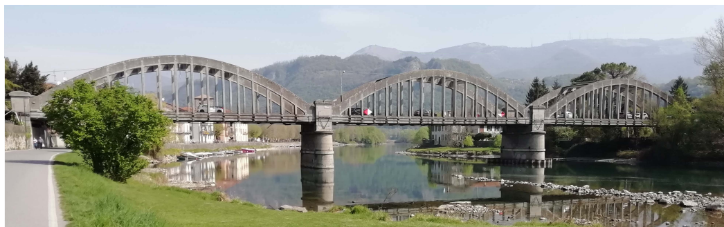
Figure 1. Brivio bridge (1917): downstream view of the road three-span arch bridge crossing the Adda river. Picture taken by author E.R. on 15 April 2022, within a period of enduring drought.
