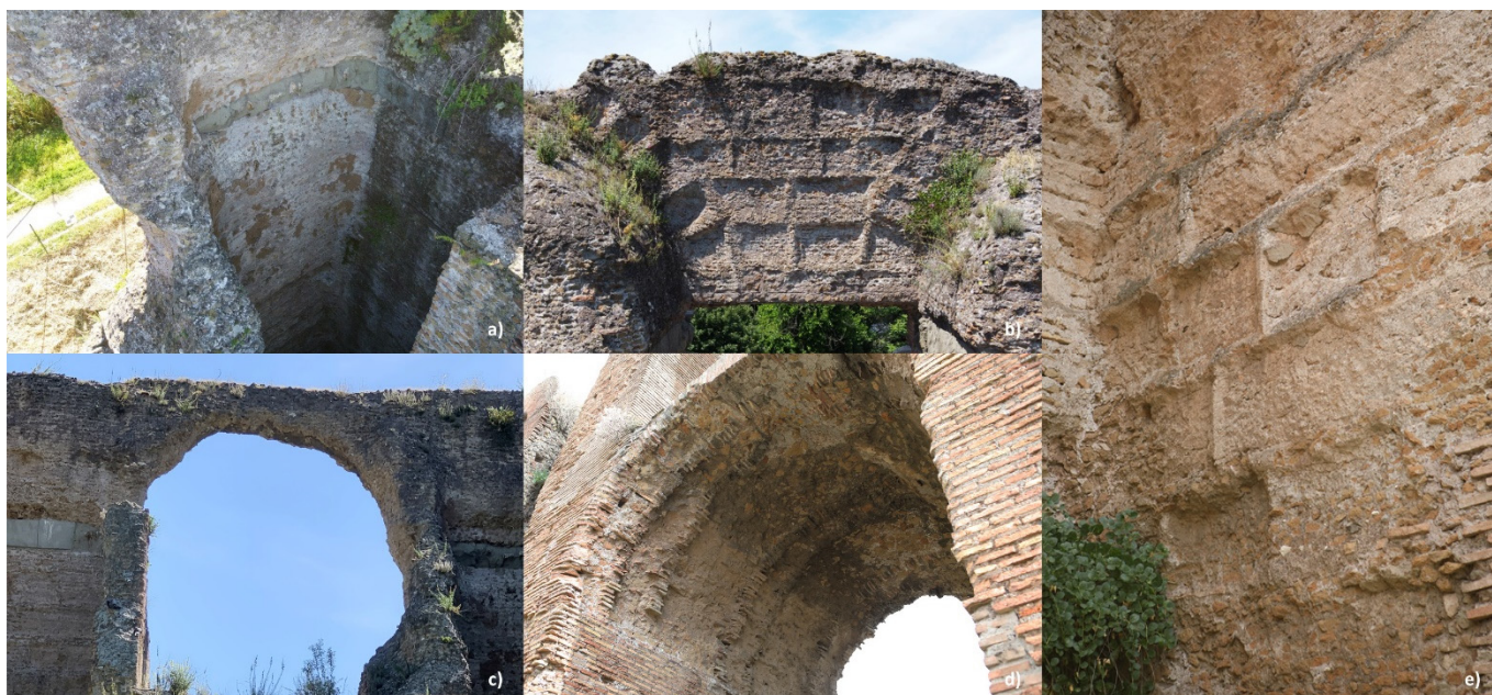
Figure 3. Section G: (a) Opus caementicium walls that were once placed all around the Claudio piers—ashlars have been removed, some traces visible on the top; (b) imprints of the peperino ashlar on opus caementicium—it is possible to recognise the square stone ashlar and the special one used for the arches; (c) opus caementicium arch—once the stones have been removed, the opus caementicium was exposed to weathering. This is an extreme case where the thickness of the arch has become thinner; (d) Hadrian structures—the arch was built with brick armchair voussoir and opus caementicium; (e) imprints of the peperino ashlars on opus caementicium.
