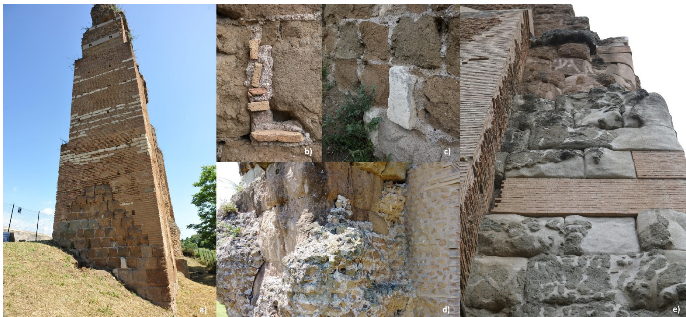
Figure 4. Section D: (a) North facade—supporting structures, base that re-used peperino ashlar stones, walls with bricks and stones courses (probably late antiquity, Honorius emperor); (b) Brick wedges to fill the mortar joints; (c) Limestone or marble among the peperino ashlars; (d) East facade—opus caementicium around the peperino piers; (e) West facade—peperino ashlar restored in 2008–2009.
