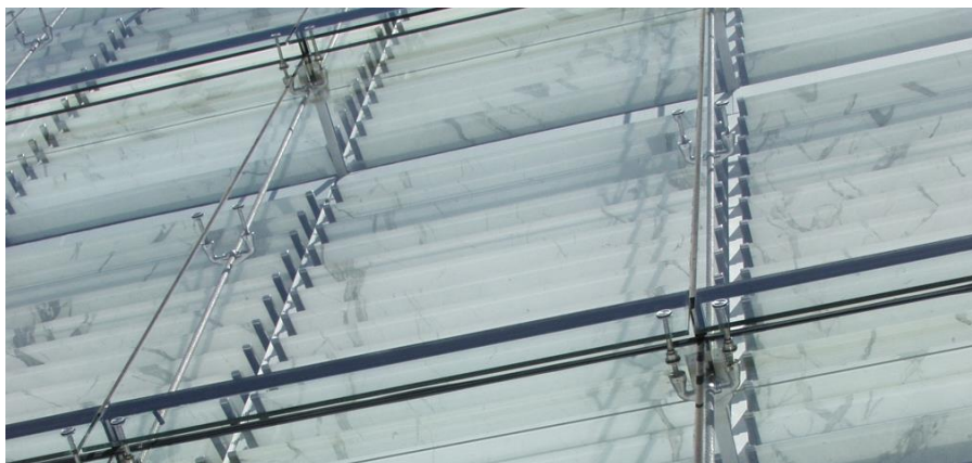
Figure 2. Integrated installation consisting of the internal curtain wall in double-glazed sheets, the cavity with sun-shading devices and the external screen in monolithic tempered glass sheets.
