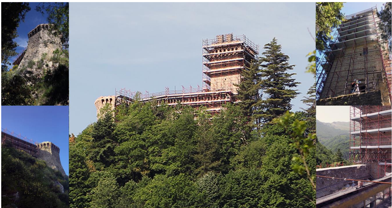
Fig. 1: The Stronghold of Arquata del Tronto with its main architectural elements after the 2016 earthquake . The bastion on the left and the tower on the right.
