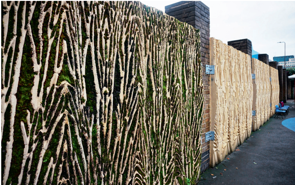
Figure 3. Poikilohydric Living Walls, installed at the St Anne's Catholic Primary School in London. Moss transplanted onto 8 bioreceptive porous TecCast panels.
