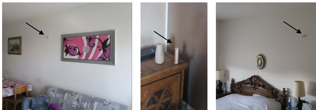
Figure 3. Sensors set up. Images from the installation in a selected apartment.
