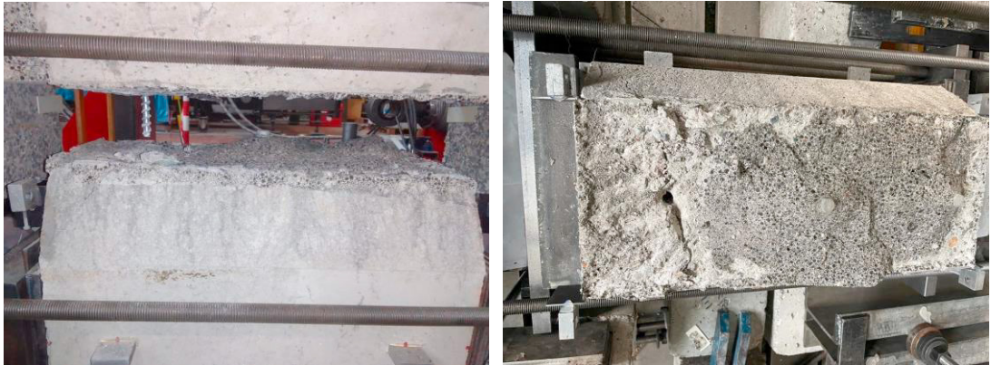
Fig. 4. Pull-out of the anchor and concrete cone failure of the overlay.
