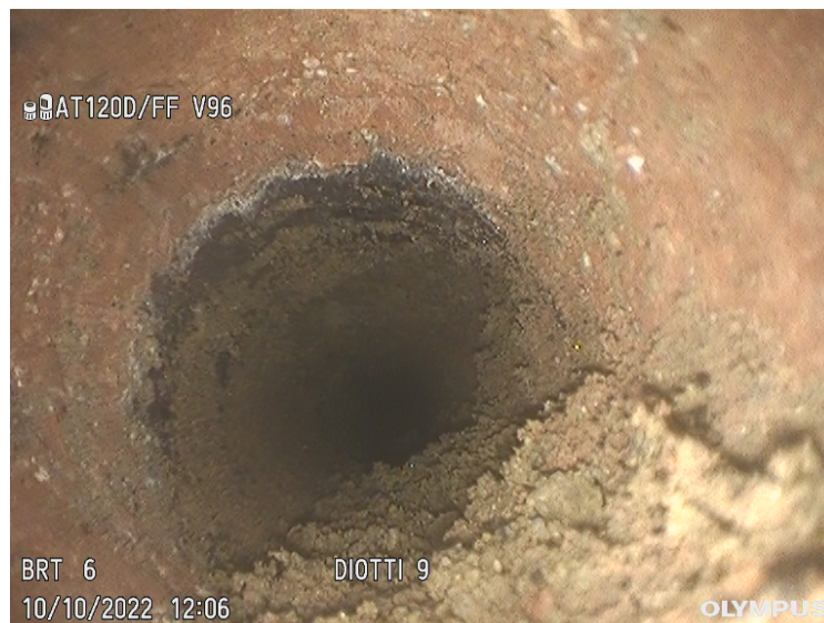
Figure 11. Image of an endoscopic test carried out in the masonry of the basement (view from the inside out). The material change between the brick and the ground is highlighted.
