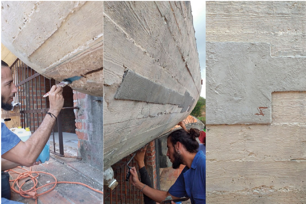
Fig. 5 Pilot site for reinforced concrete's restoration. Courtesy of Assorestauro, photo by Davide Del Curto
