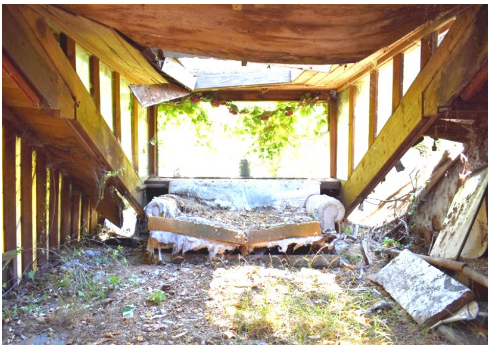
Figure 9. Collapsing and decomposing structures at Druid Heights (2020) Photograph by the author
