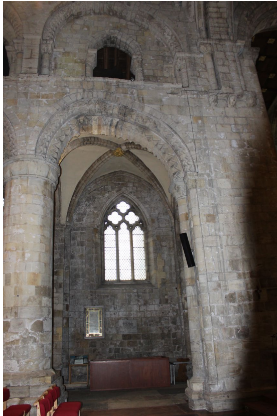
Figure 7. Visible deformation at Selby Abbey
