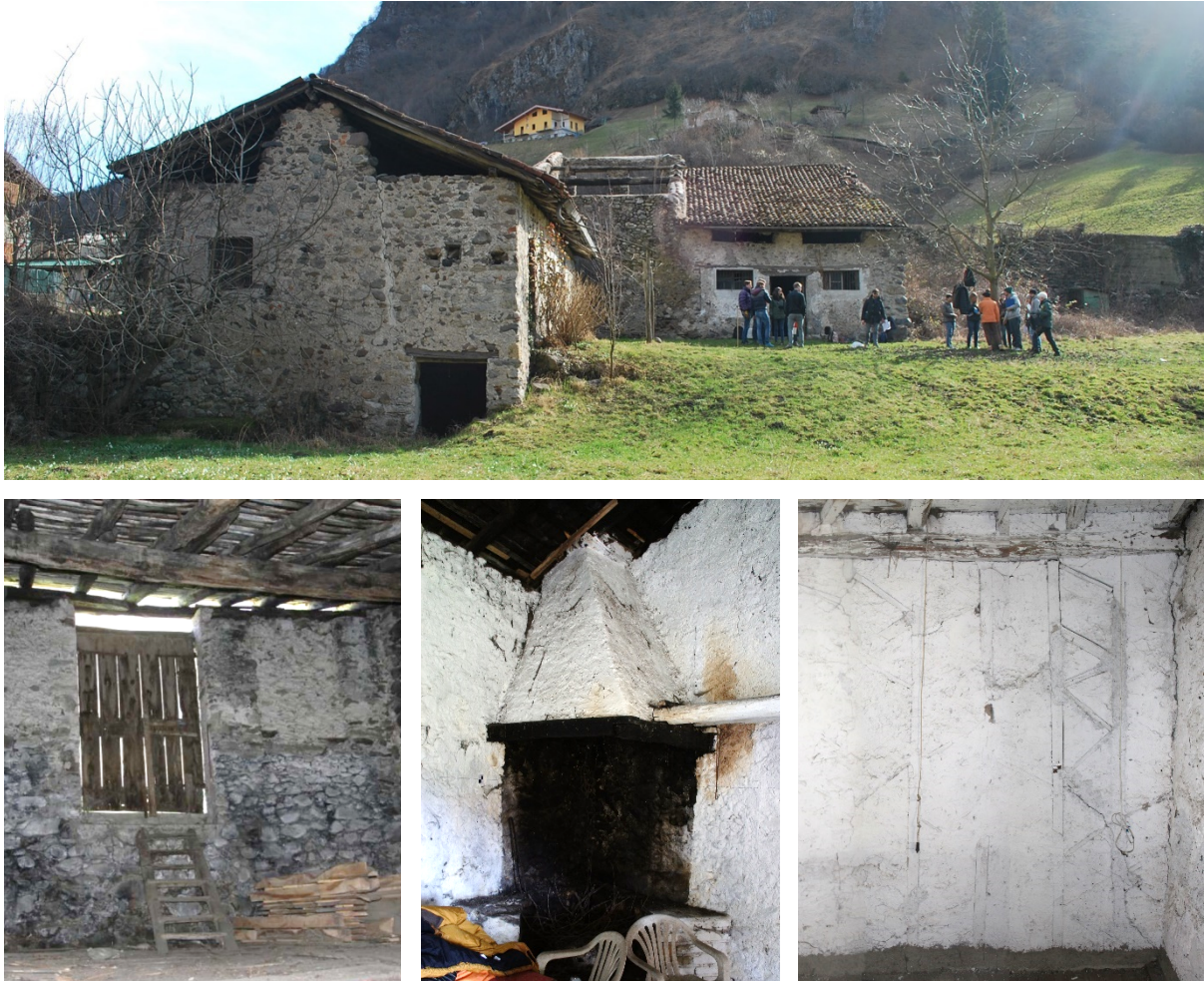
Figure 1 – General photo of the two rural buildings of the Rebecco Farm complex during a survey phase with students. At the bottom building A, where you can see that the roof is maca in some rooms; on the left, building B.
