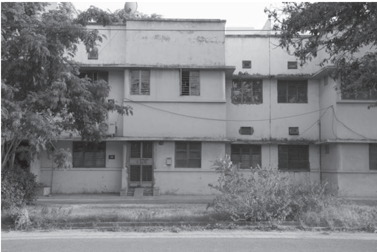
Figure 3.23 Photographs of a Group of Houses in RK Puram Colony, 2014 Source: Author.
