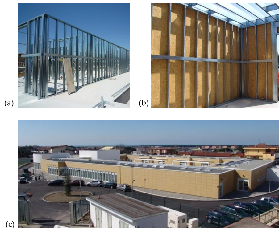
Figure 1. CFS school construction process: (a) CFS structural walls, (b) Sheathing of CFS walls, and construction of the roof, (c) Finishing and final result.
