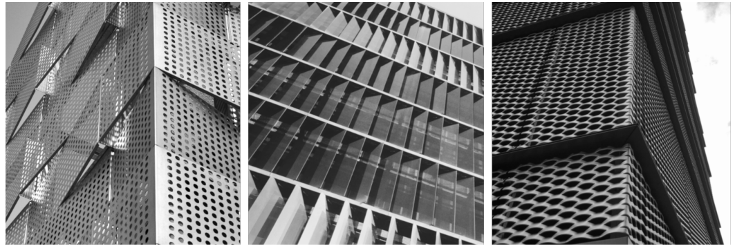
Figure 1. Permeable screen types on building facades: perforated screens, louvers, expanded mesh (left to right).
