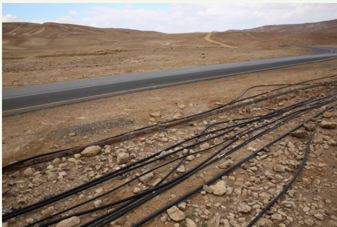
Figure 5. Black pipes in the 'Negev', 2020. Photographed by Dan Farberoff.
