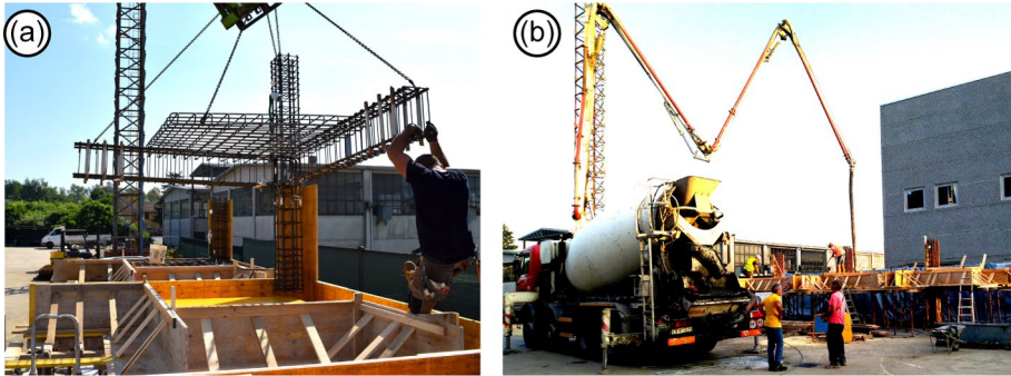
Fig. 6 Corner joint specimen: a formworks and reinforcement cage; b casting operation. (Note. The Reader is referred to the color version of this figure)
