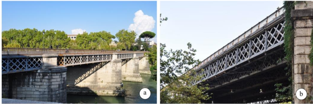
Figure 1: Palatino Bridge, Italy: (a) Southside of the bridge; (b) Truss beams of the deck.
