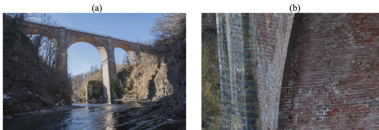
Figure 1. The Olla bridge: (a) picture from the Stura River; (b) existing damages on the second arch.
