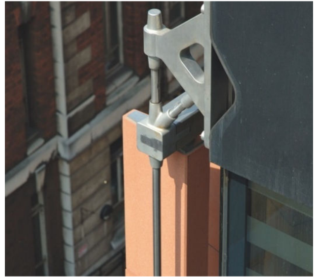
Fig. 29. Nicholas Grimshaw and Partners, UCL Cancer Institute , London (©Courtesy of Sannini Project).
