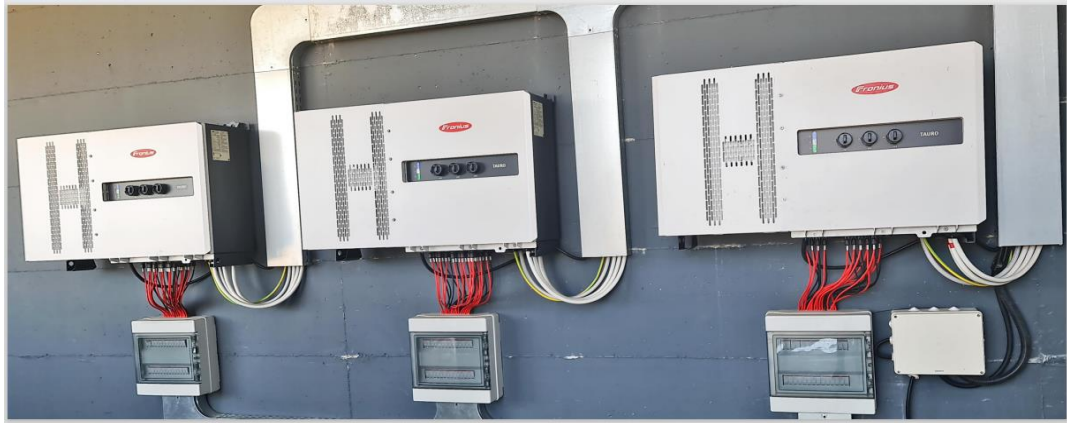
Figure 2: View of the inverters installed in the object.
