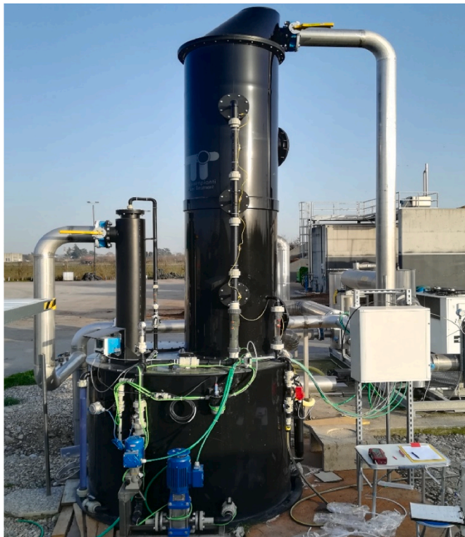
Fig. 2. Absorption column of the plant.
