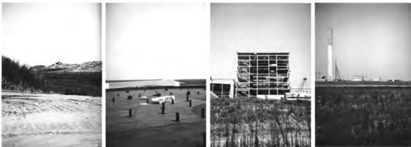
FIGURE 14.10 Photographs taken during the construction of the Porto Tolle power station: (a) transport of sand to the southern part of the site, aimed at preparing the ground of the future oil depots; (b) an oil depot in the northern area of the site and the Po River entering the Adriatic Sea; (c) the machinery hall and the boilers; and (d) the chimney, oil depots, and piling rigs. Source: Vinicio Zanardi.
