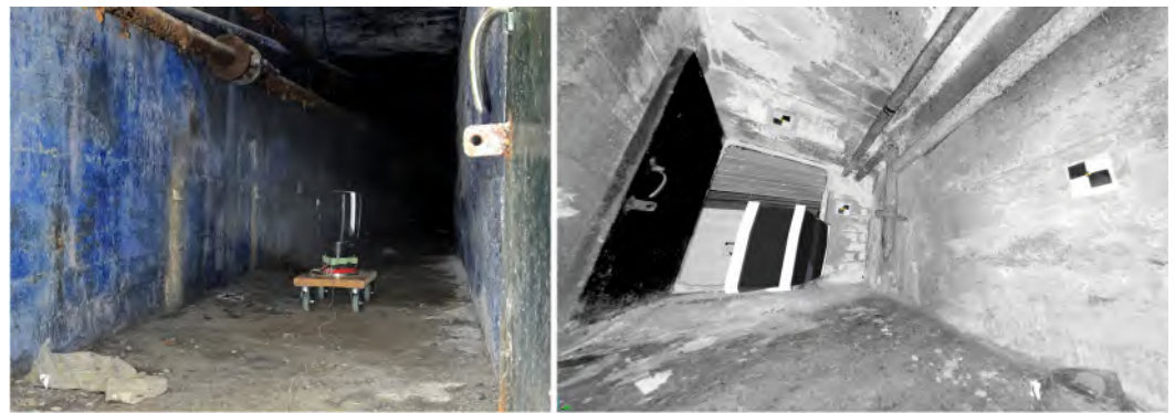
Figure 5. The laser scanning acquisition of the tunnel used in the second lab experiments.
