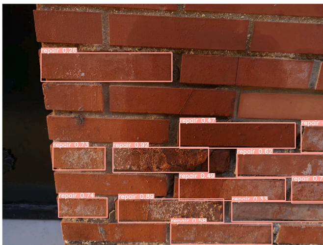
Fig. 8. Test to visually check if the algorithm responds correctly, especially in “repair”.
