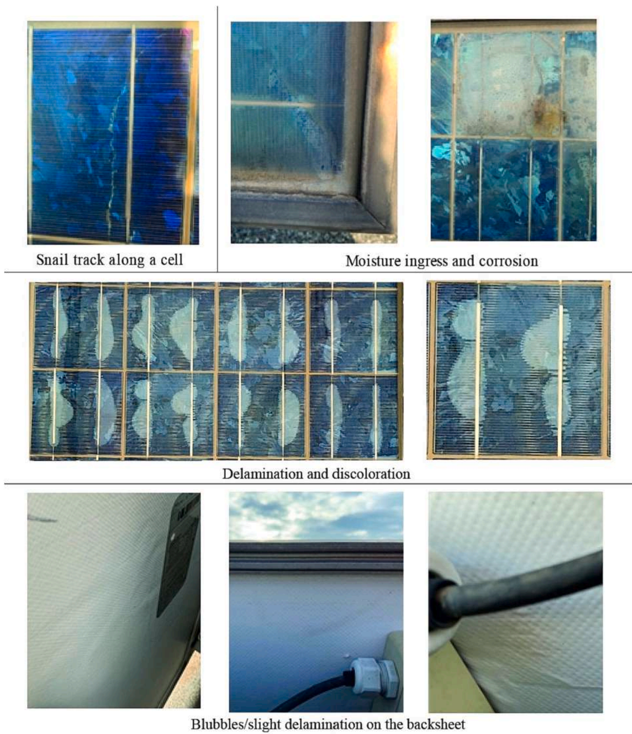
Fig. 9. Overview of the main detected alterations.
