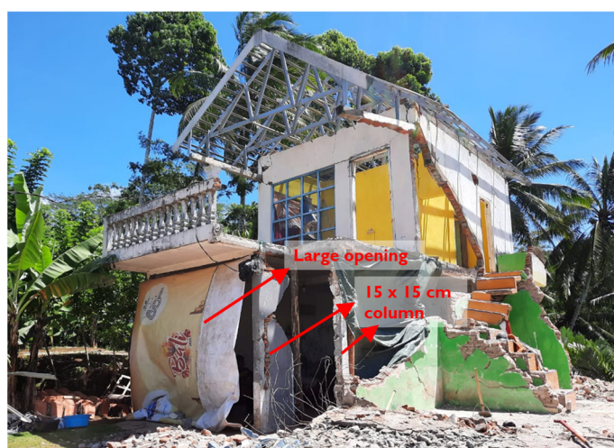
Figure 1. Heavy damage on a two-story confined masonry (CM) with a large opening and substandard RC frame.
