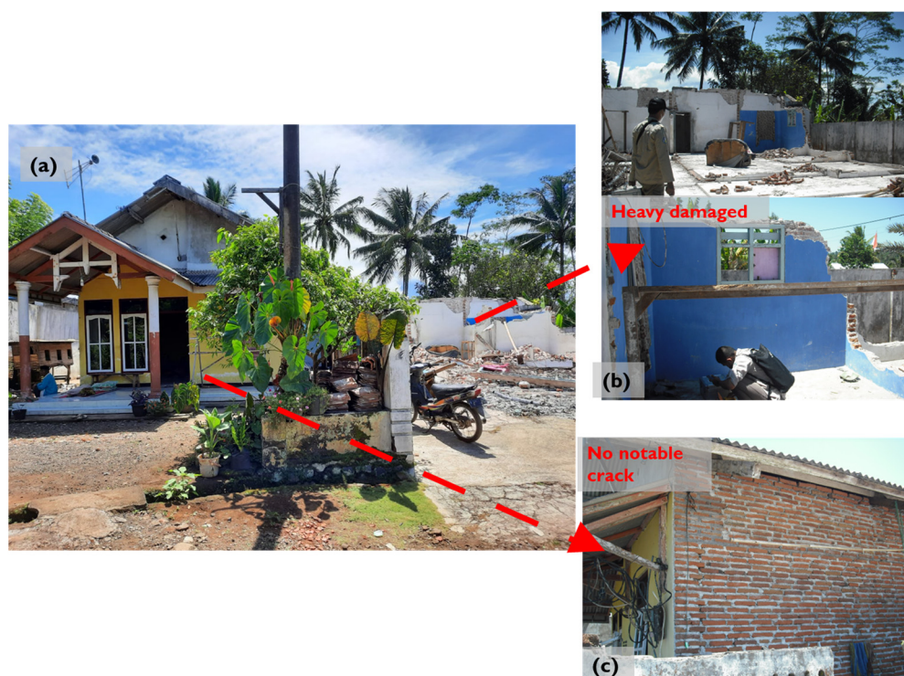
Figure 3. (a) Two neighboring UM housing after an earthquake: (b) heavy damage on the right house, while (c) no remarkable damage on the left house.
