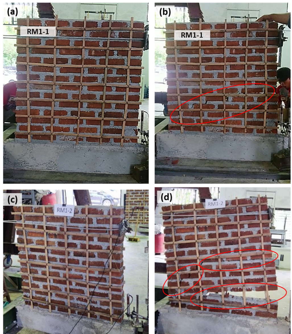
Figure 17. The pushover shear test and crack patterns of the retrofitted masonry panels with 2.88% of bamboo retrofitting: (a,b) RM1-1, and (c,d) RM1-2.
