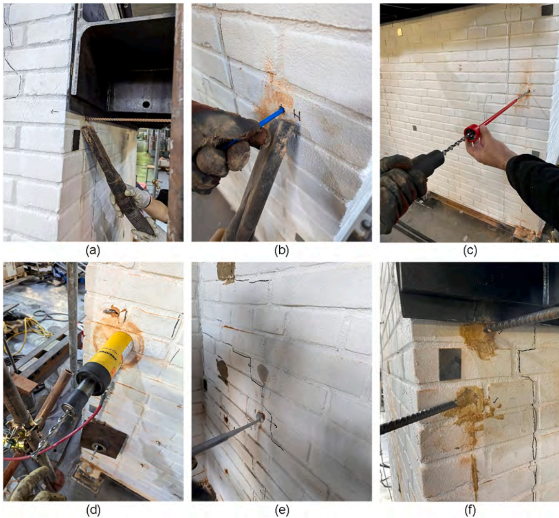
Fig. 4. Retrofitting steps: (a) hole drilling, (b) compressed air cleaning, (c) twisted bar installation, (d) twisted bar removal, (e) adhesive injection, (f) rebar installation.
