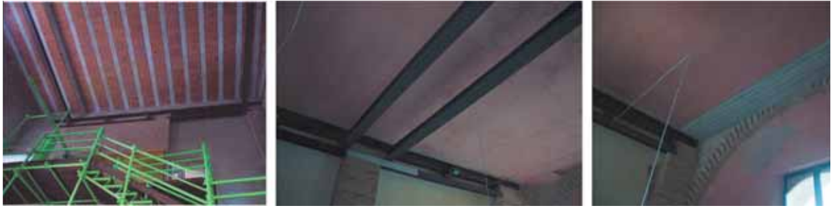
Fig. 4. Two couples of steel beams are present in each room situated on the longer arm of the Castle; one couple runs along opposite walls and the other is aimed at linking the first two beams.
