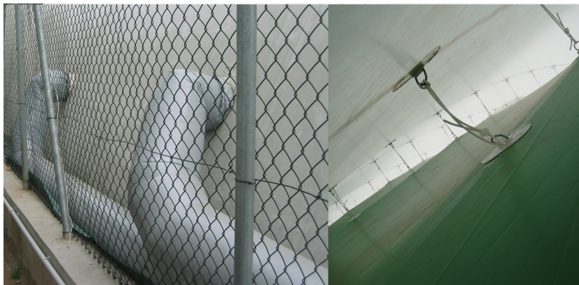
Fig. 7. 3rd generation sport hall: ducts for the air flow rate into the air gap between the two envelopes (left) and view of the air gap between two membrane layers (right).
