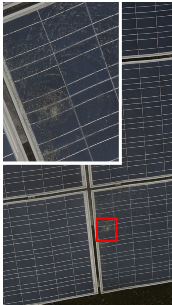
Fig. 9. Picture captured by a Nikon1-v1 camera with inlet detail of a particular shock-defect.
