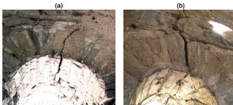
FIG. 4. Details of the passing-through cracks at the keystones of the arched openings.
