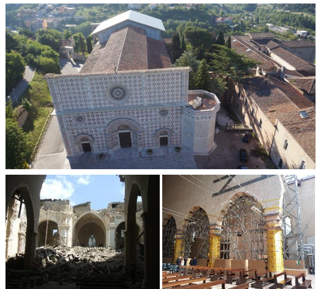
Figure 2. Top: an image of the Basilica acquired with the UAV platform AscTec Falcon 8. Bottom: on the left an image of the transept area immediately after the earthquake in 2009. On the right the consolidation structures to strengthen the octagonal pillars of the naves (2012).
