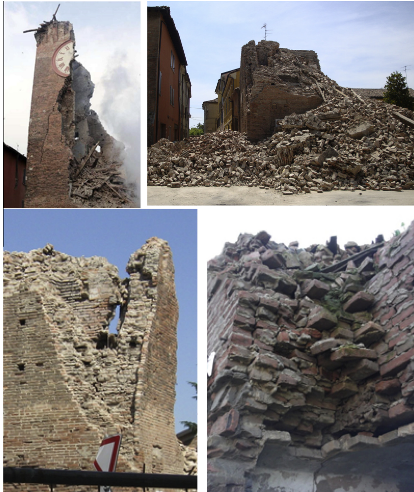
Fig. 1. Meaningful images of the survived part of the tower after the 20th May seismic event.
