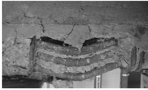
Figure 13. Plastic hinge at mid span of beam No. 5.
