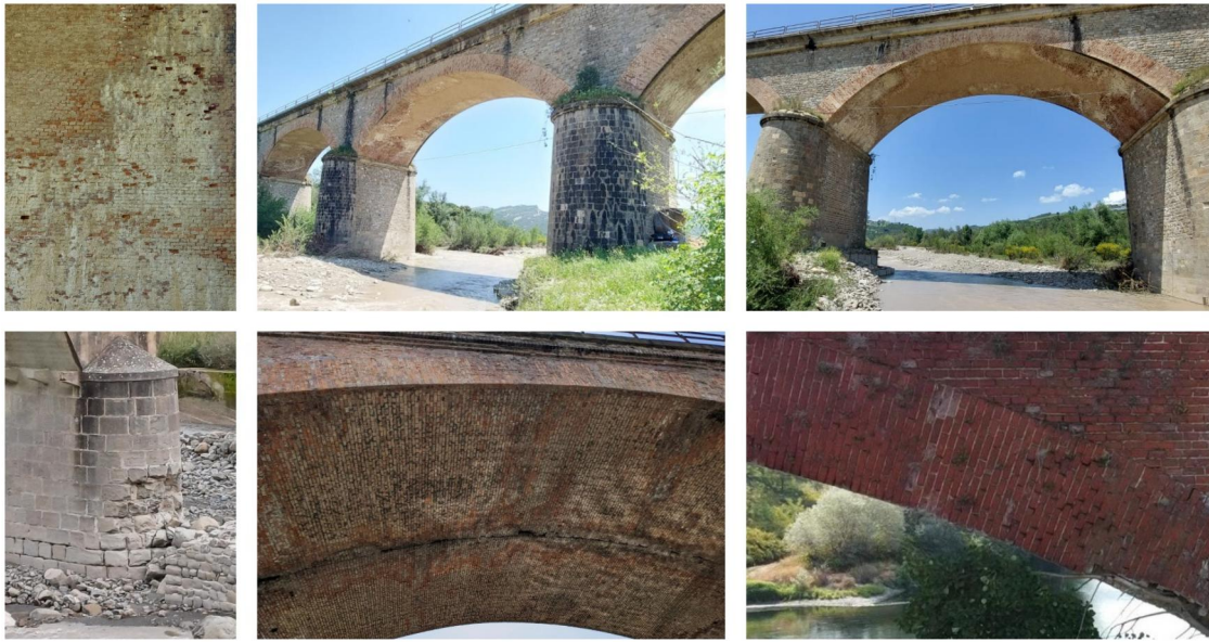
Figure 1. Typical defects and critical issues that can be found in real case studies (from top, left to bottom, right): environment agents-induced degradation and material voids; impact damages and erosion; longitudinal cracks.
