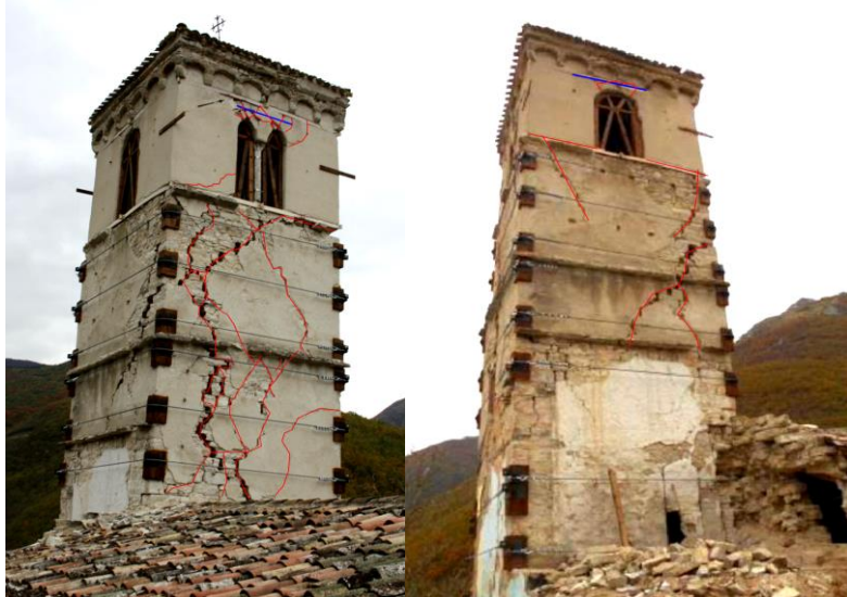
Figure 7. Damage to the bell tower: west and east side (Da Porto & Modena, 2020).
