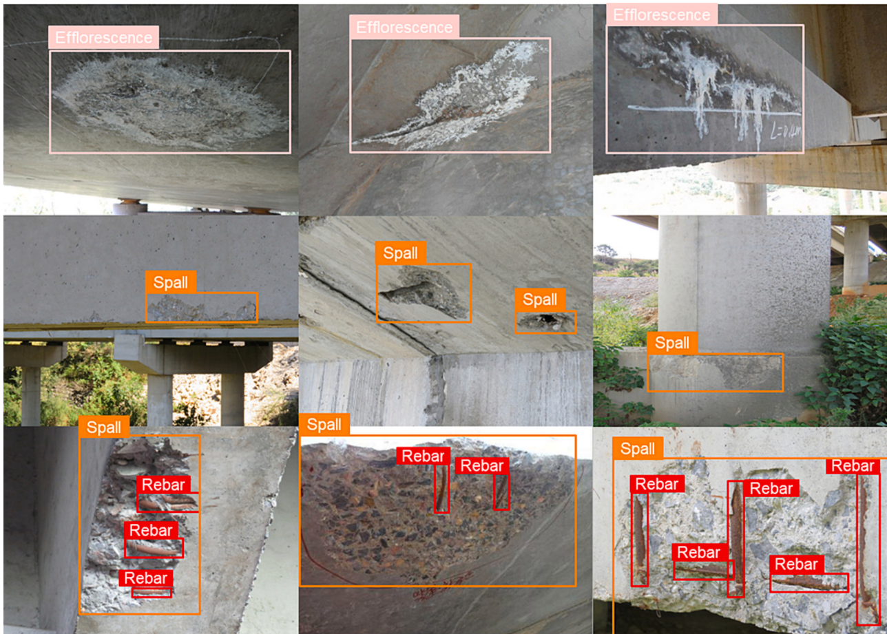
Fig. 7. Examples of different types of annotated defect images in the concrete bridge damage dataset [104].
