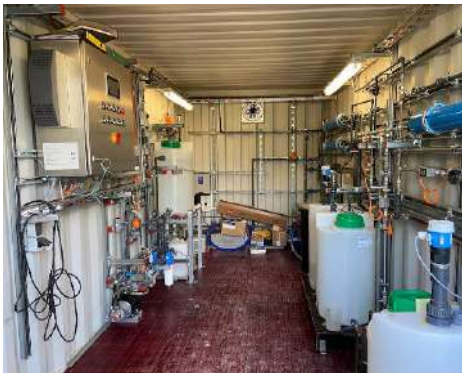
Nanofiltration and reverse osmosis desalination system
