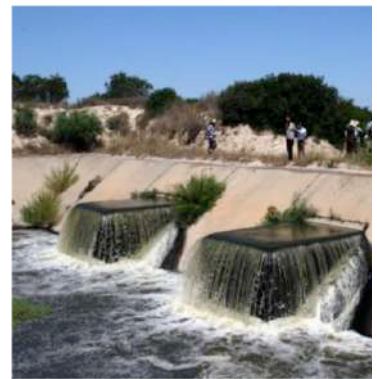
ONAS wastewater treatment plant
