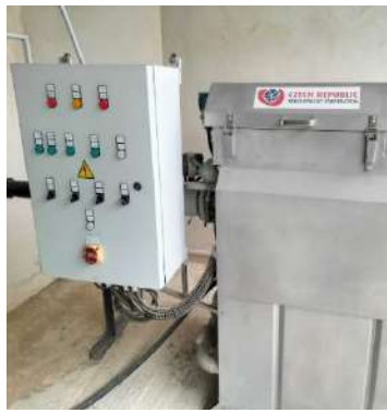
UV wastewater treatment system
