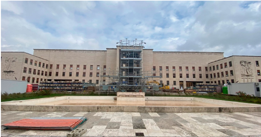
Fig. 2 The huge construction site recently installed at the heart of Sapienza’s university campus (photo Salvo, February 2024)
