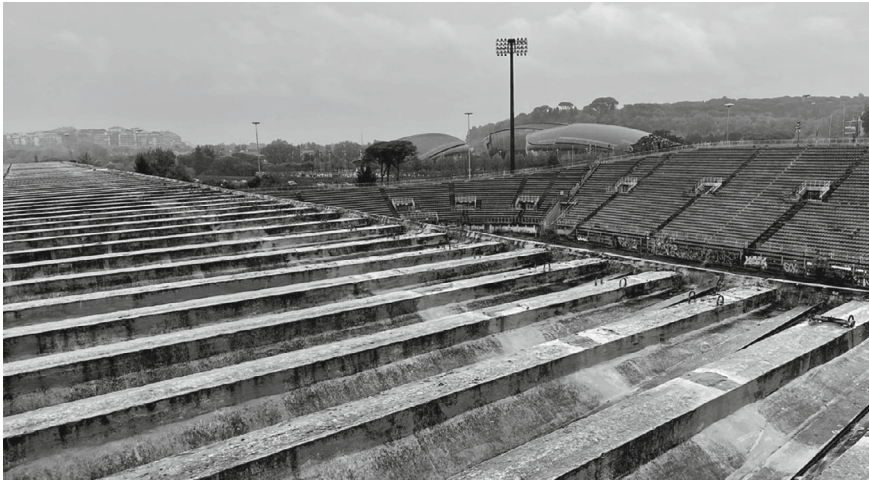
Fig. 4 Ferrocement cantilevered roof after improper lighting and loudspeakers devices removal
