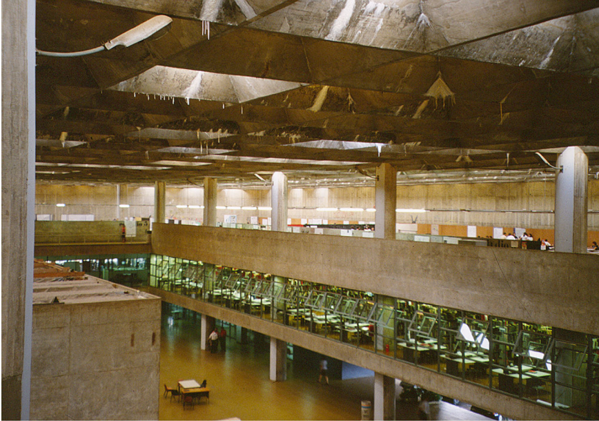
Fig. 3 Vilanova Artigas building: infiltrations, 2002 (Photo Beatriz Kühl)
