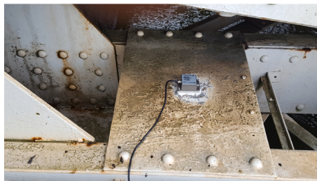
(a) Inclinometer placed at bridge support.
