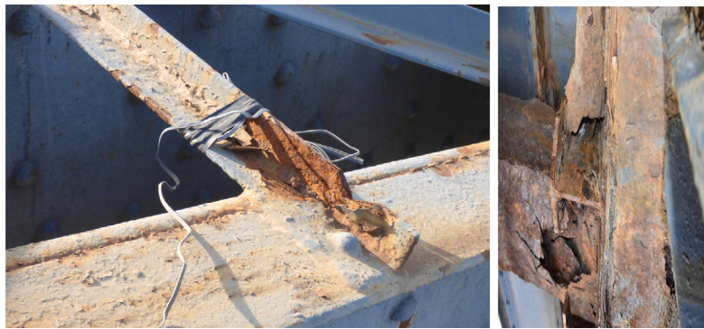
Fig. 1. Local corrosion of steel elements (original figures not related to the case study).
