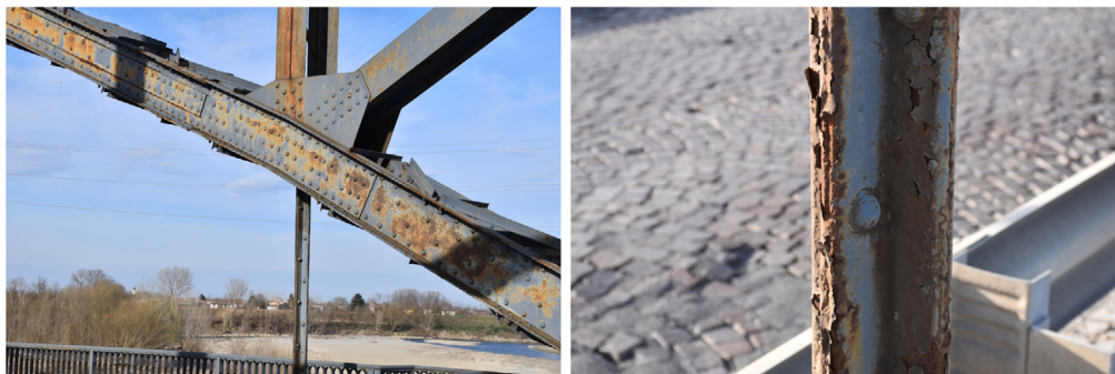
Fig. 2. Corrosion through a whole steel element (original figures not related to the case study).
