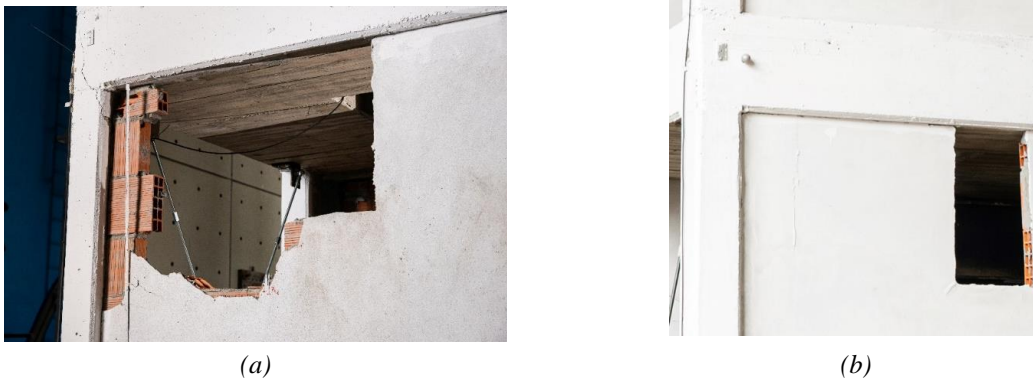
Fig. 4 - Detailed view of a selected region of the Buildings: a) cracking of the column-slab joint region of the first floor in Building A, b) column-joint region of Building B with no signs of distress.
