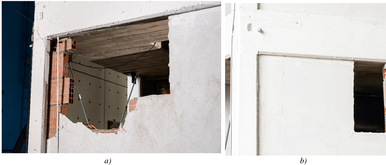
Figure 10 – Detailed view of a selected region of the Buildings: a) cracking of the column-slab joint region of the first floor in Building A, b) column-joint region of Building B with no signs of distress.
