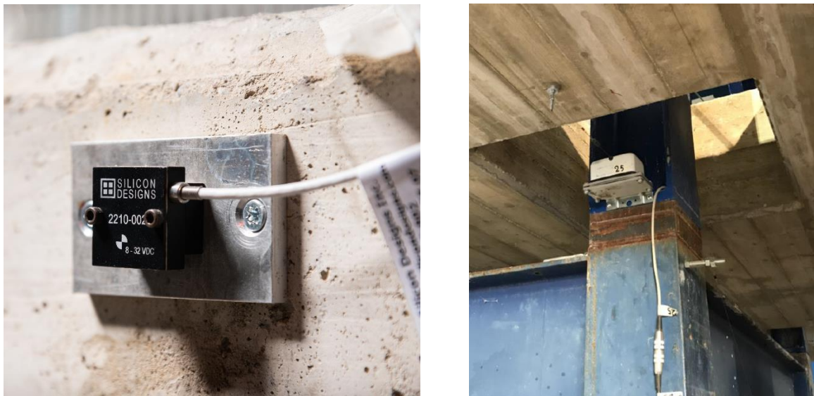
Figure 6 – a) View of installed accelerometer sensor; b) View of installed displacement transducers
