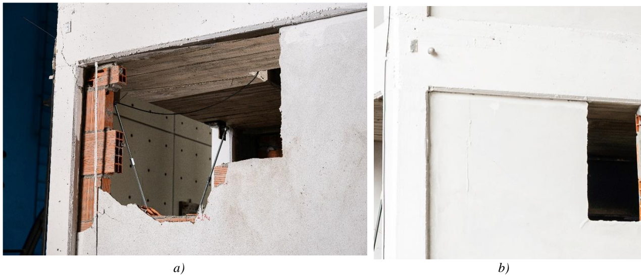
Figure 10 – Detailed view of a selected region of the Buildings: a) cracking of the column-slab joint region of the first floor in Building A, b) column-joint region of Building B with no signs of distress.
