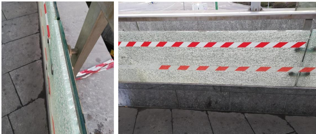
Figure 1. Fractured laminated tempered glass in Italy.
