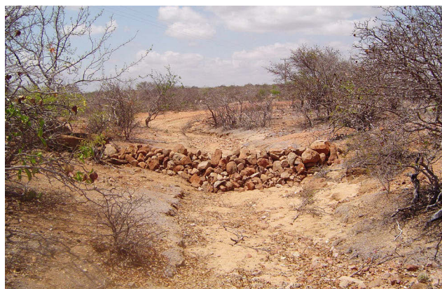
The dike is a permeable wall built in an ephemeral stream. Photo: P Barretto
