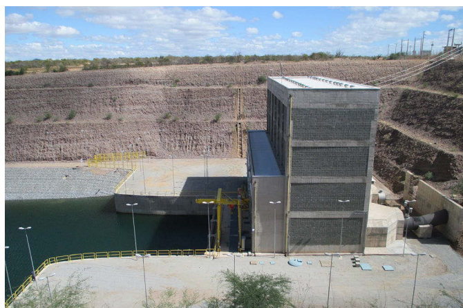
The first water withdrawal and pumping station of the water diversion project (eastern channel system, Itaparica Reservoir). Photo: M Siegmund-Schultze
