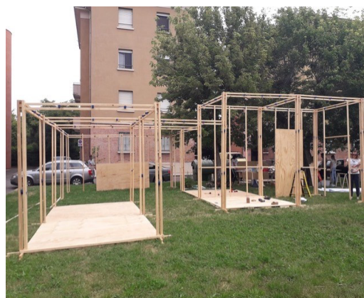
Fig. 3 Phase of construction of temporary structures to verify the effects of the reorganization of public spaces in the Living Lab experience “Rigenerare il Ciano”.
