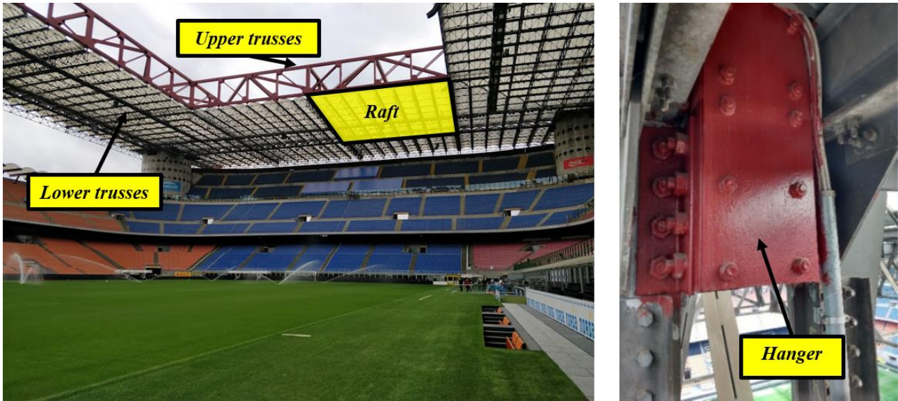
Figure 1 The steel roof of the G. Meazza stadium (left) and a detail of bolted joints connecting upper and lower trusses (right)
