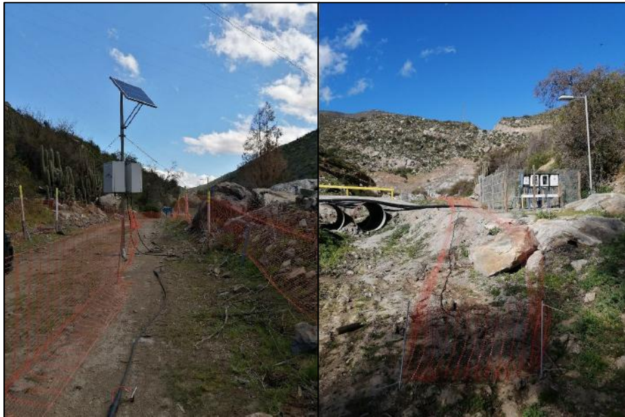
Figure 1 G.Re.T.A. system installed downstream the tailings dam in Chile, Profile 1
