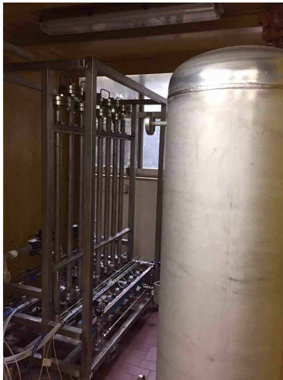
FIG. 28. Test plant used for characterizing and selecting sorbents for the UAr extraction plant PSA unit.
