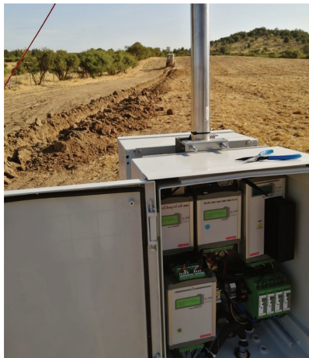
Figure 5 G.RE.T.A. installation in Chile: the measuring box (foreground) and the trench (background)
