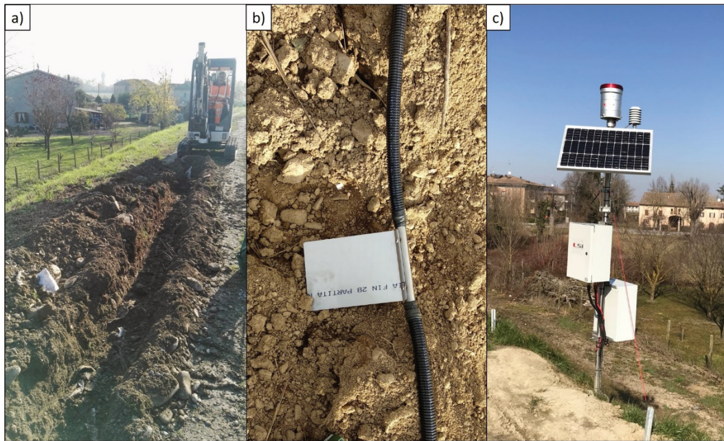
Figure 4 G.RE.T.A. installation in Colorno: (a) Trench on the top of the levee; (b) Protected cables and plate electrode; (c) Geo-resistivimeter and meteorological station boxes
